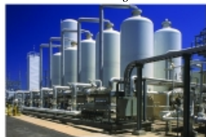
From drilling rigs to refineries; from processing control to hazardous material storage
